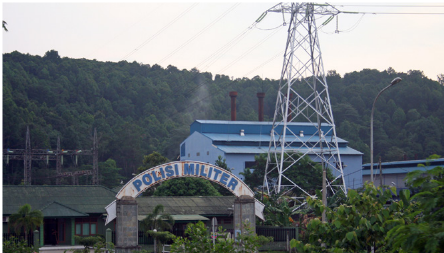
Military Police base with what appears to be their own power plant in Batuampar, Indonesia (photo credit: Vetatur Fumare (CC BY-SA 2.0)).
