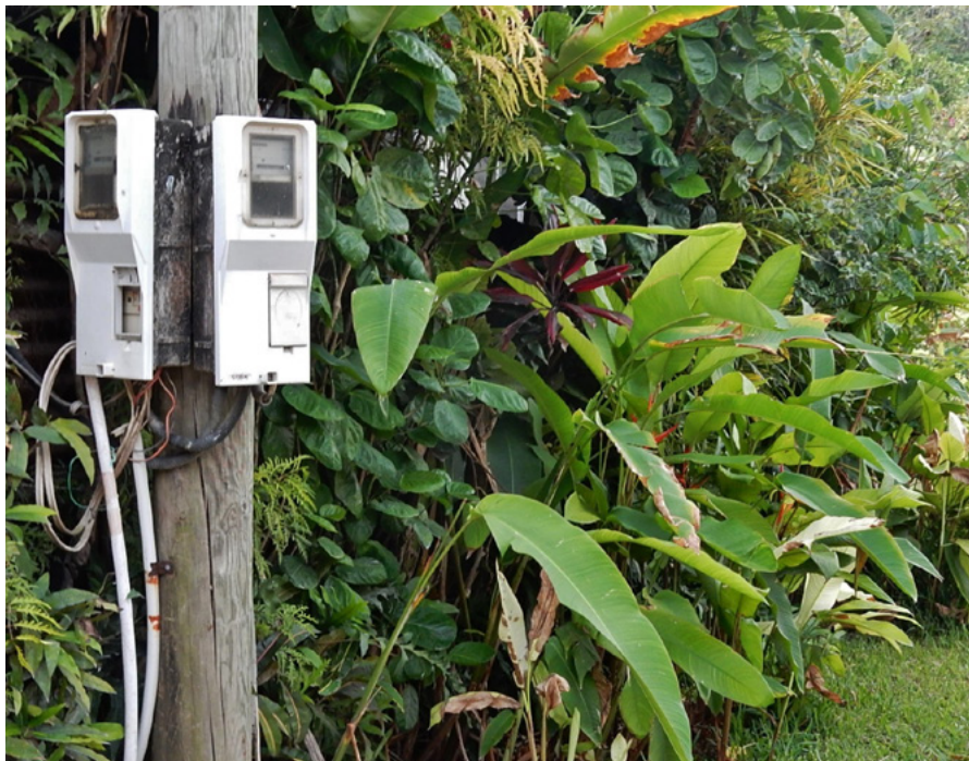
Power meters are surrounded by lush vegetation in Luganville, Vanuatu. (Photo credit: Michael Coghlan, CC BY-SA 2.0).
